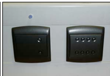
Custom control panels to power up amplifier rack, projectors and screens
